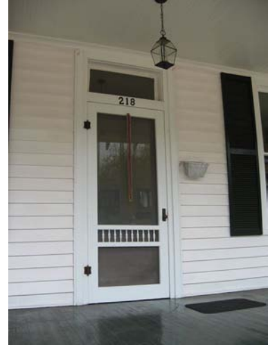
An appropriate screen door at 218 K Street does not conceal the original wood door behind it.
