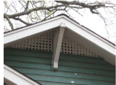
Trim such as eave brackets should not be removed or concealed (1015 N. 5th Street).
