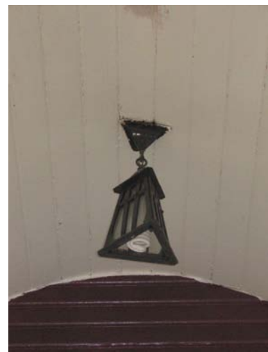
Over-head hanging light fixture at 406 Auburn Avenue.
