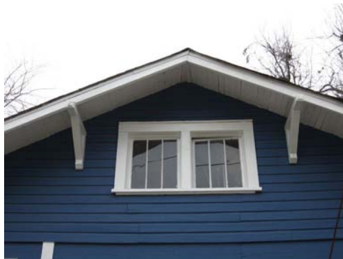
Several architecture styles may include wooden eave brackets that could become deteriorated by a leaking roof. These at 417 Park Avenue are well maintained.
