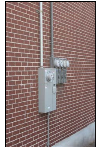
These meters are correctly placed on a non-primary elevation.
