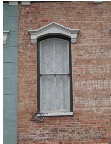
Original two-over-two wood sash window with ornamental hood at 120 S. Grand Street.
