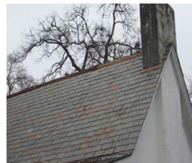
The slate roof at 1005 S. Grand Street is a unique historic element that should be preserved. Maintenance is more cost effective than replacement in kind.
