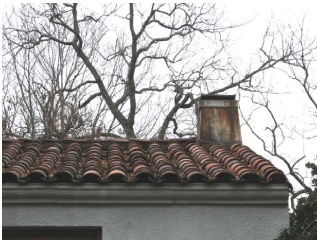
The clay tile roof at 1204 St. John Drive helps define the historic character of the dwelling.
