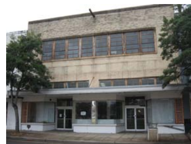
The original transom above the 1950s storefront at 117 Desiard Street is intact and not concealed.
