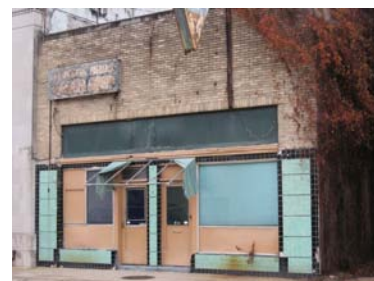
The transom at 103-105 Catalpa Street could be uncovered as part the of building's restoration.
