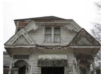
The highly decorative features of the Roland Filhoil House should be repaired as needed and re-painted to preserve this distinctive dwelling.
