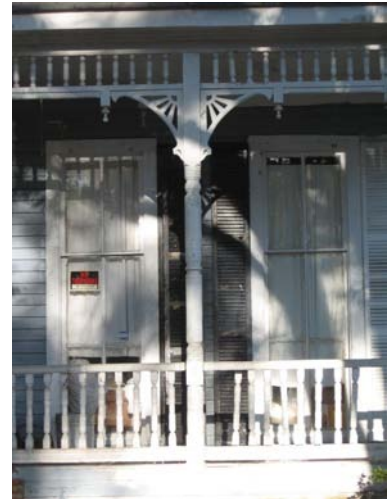
Porches like this one at 1205 St. John Street often have an abundance of wood elements, including milled posts, railing and balusters, and ornamental trim.
