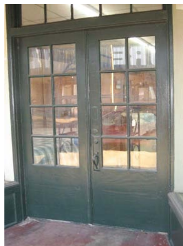
Original doors should be preserved and maintained such as at 504 Desiard Street (above) and 131 N. 2nd Street (below).
