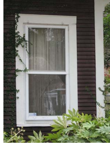
Storm windows like at 406 Auburn Avenue protect original windows and provide an insulating effect that make retaining historic windows more cost effective than replacing them.
